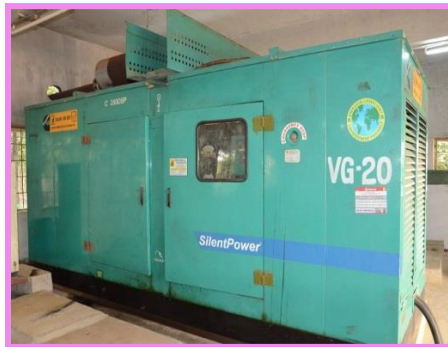
Power Back Up (150 KVA)
